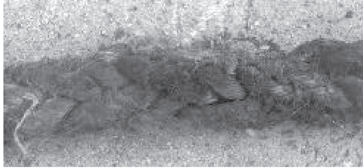
Figure D-006 Extensive External Abrasion
